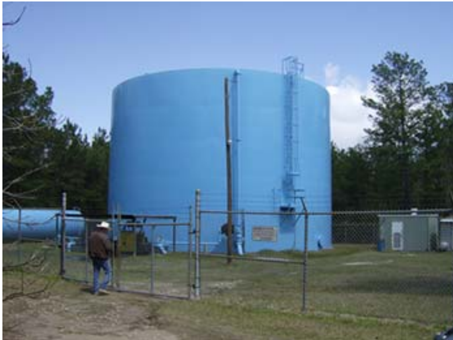
Waterwood MUD Storage Tank
